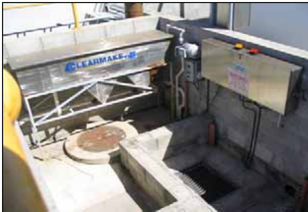
Oil / Water Separator Mooloolah River Fisheries
