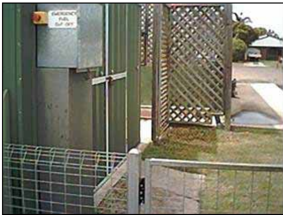
Emergency Fuel Shut-off Kawana Waters Marina
