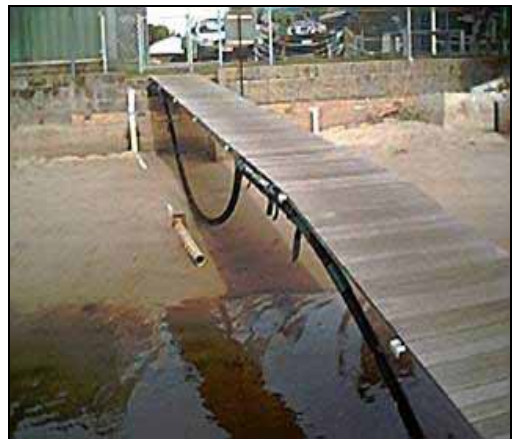
Fuel Line to Dock Kawana Waters Marina
