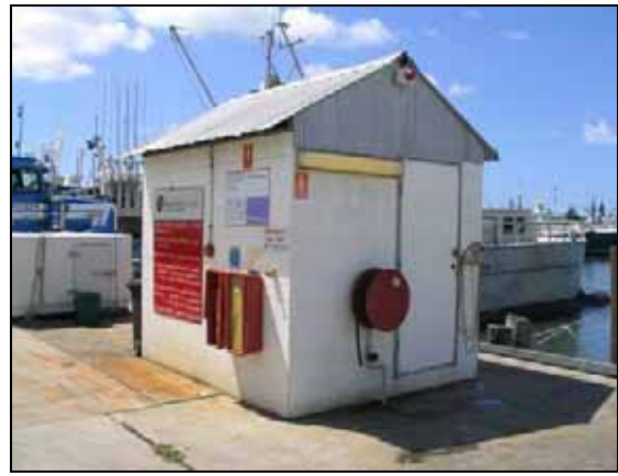
Emergency Fuel Shut-off Browns Main Wharf
