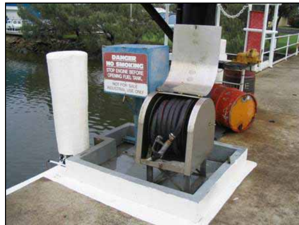
Refuelling Hose Reel Mooloolaba Pilot Station
