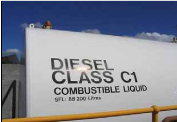
88,200 Litre Fuel Storage Tank Mooloolah River Fisheries
