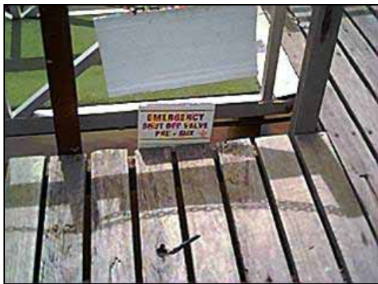
Emergency Shut-off Valve 1 ‘O’ Boats
