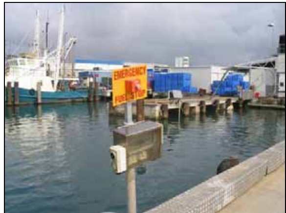
Emergency Fuel Shut-off at the 6 Fuel Outlets De-Brett's Wharf
