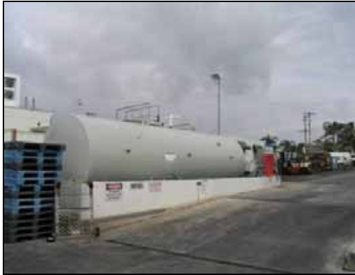
56,000 Litre Diesel Fuel Tank De-Brett's Wharf
