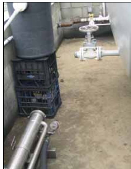
Diesel Tank Oil / Water Separator De-Brett's Wharf
