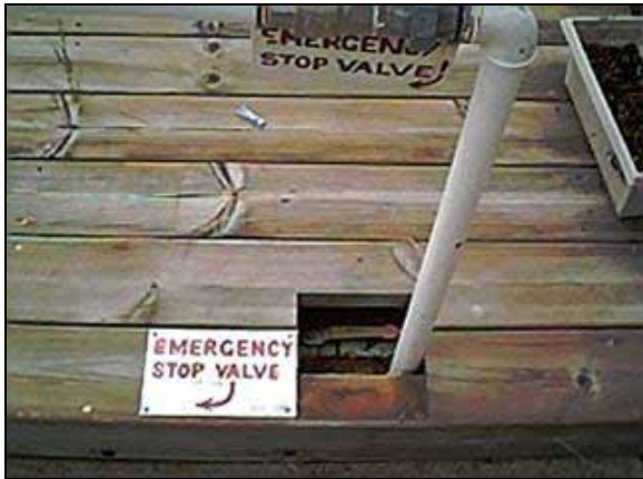
Emergency Shut-off Valve 1 Pelican Boat Hire
