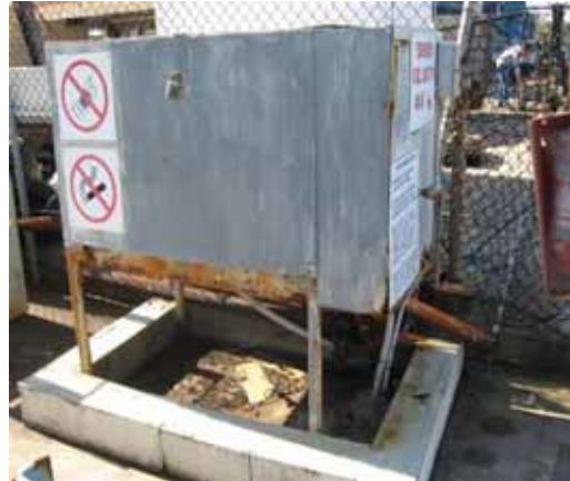
Diesel Fuel Outlet (not in use) Tabuka Wharf
