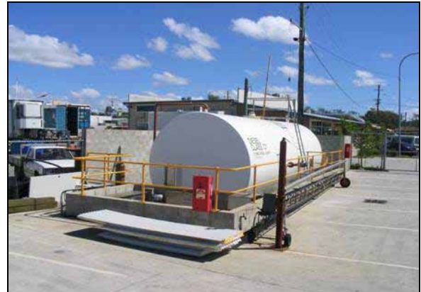
88,200 Litre Fuel Storage Tank Mooloolah River Fisheries
