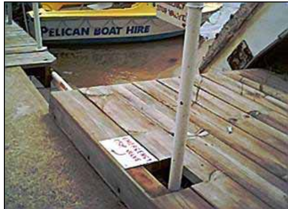
Emergency Shut-off Valve 2 Pelican Boat Hire
