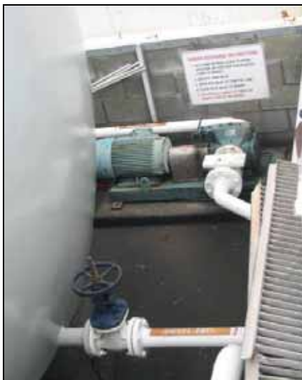
Diesel Tank Outlet & Pump De-Brett's Wharf
