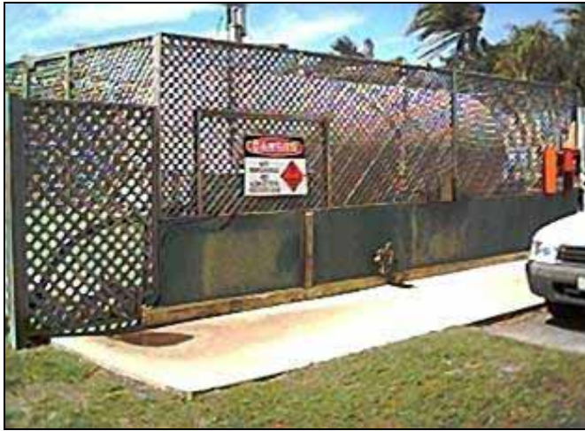
20,000 Litre Diesel Fuel Storage Tank Kawana Waters Marina
