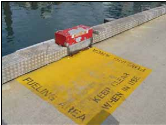
Close up of the Fuel Outlets De-Brett's Wharf
