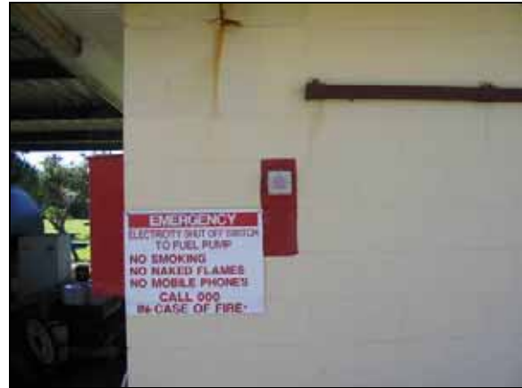
Emergency Shut-off Switch Mooloolaba Pilot Station
