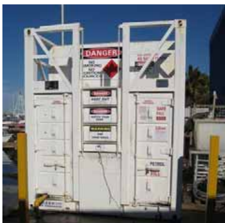
ULP/Diesel Storage Container (12500 litre) Browns Slipway
