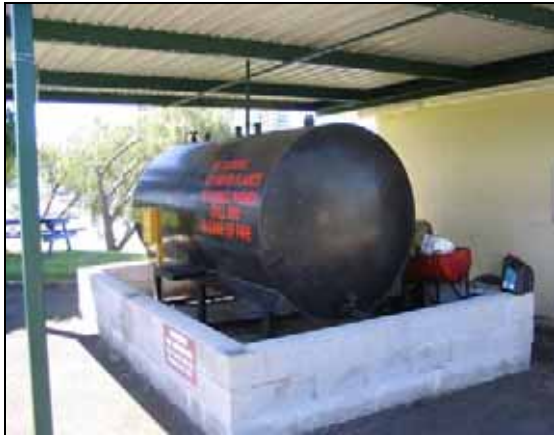
5,000 Litre Diesel Fuel Tank Mooloolaba Pilot Station
