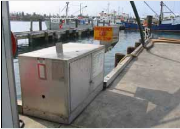
Fixed Bowser Cabinet & Emergency Stop De-Brett's Wharf
