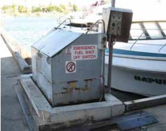
Diesel Fuel Outlet Tabuka Main Wharf
