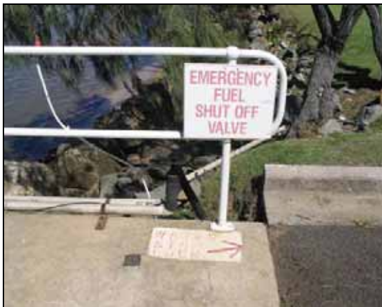
Emergency Fuel Shut-off Valve Mooloolaba Pilot Station
